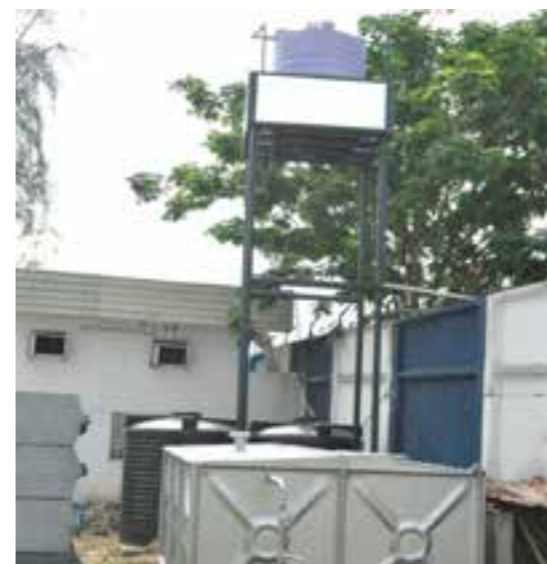
Water treatment plant at Nigerian Navy Hospital, Victoria Island, Lagos executed by our Human Resources Division
